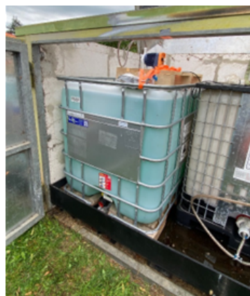
Dosing tank with ready-to-use solution
