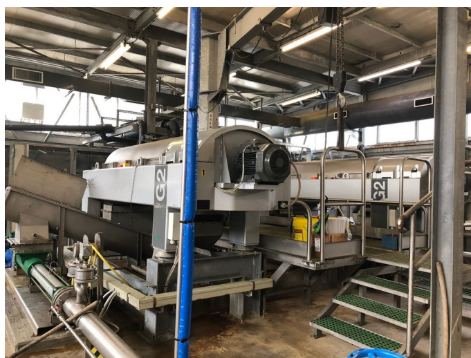
Photo 3 — Dewatering room: decanter centrifuges and cake removal by screw conveyor. The product arrives here with the polymer, without any modification of the line.
