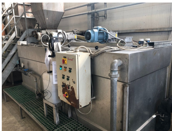
Photo 1 — Polymer preparation unit. The dosing pump and the product canister are simply placed at the foot of the unit, next to the control cabinet.
